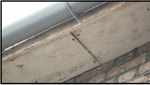
Asbestos Soffit Board
