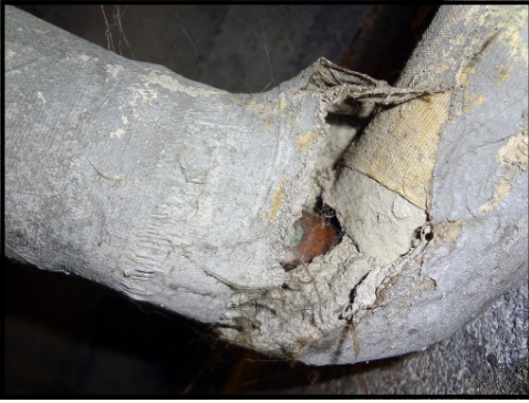
Asbestos Pipe Insulation
