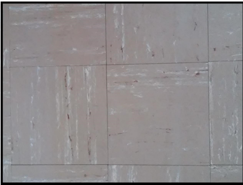
Vinyl Floor Tiles with Asbestos
